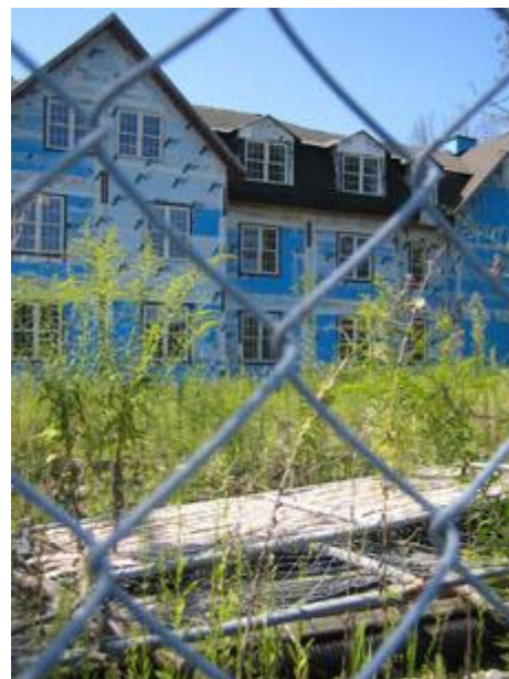
[ Media Credit: Alex Seise ] The partially finished apartments on Metzger Drive are scheduled for demolition.
