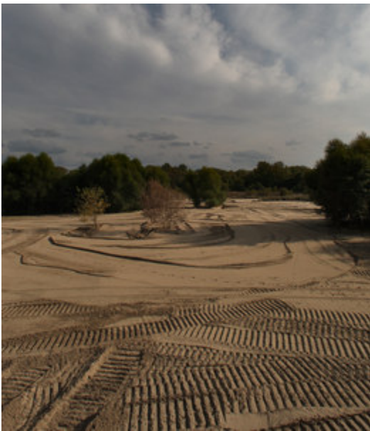
DAVID M WARREN / Inquirer Staff Photographer Tons of muck pulled from the Delaware in a controversial dredging project cover about 10 acres of the Palmyra Cove Nature Park.
